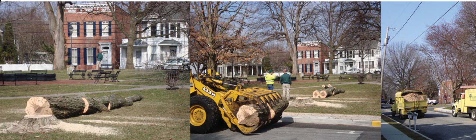
Local contractor Bartlett Tree Experts and City of Westminster Public Works staff worked together in March 2009 to safely remove several old
