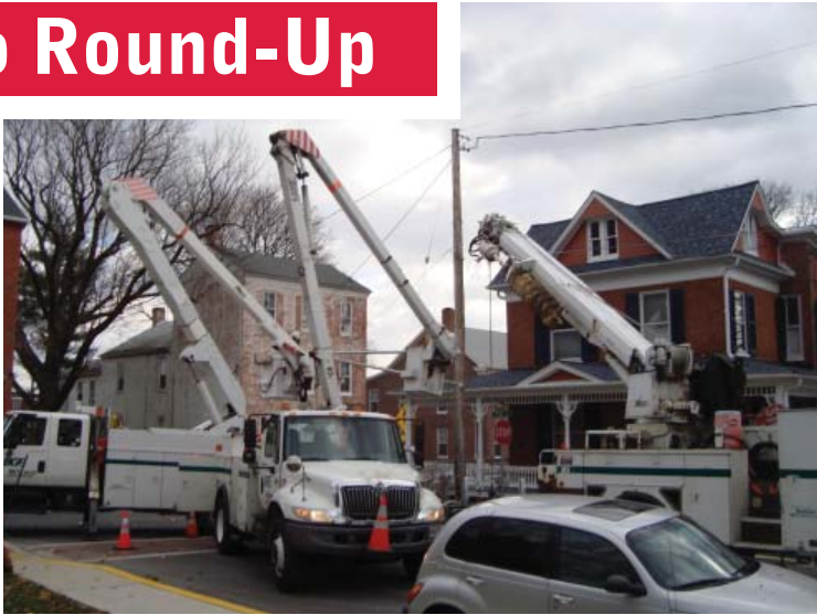
Power and utility poles are in the process of being repaired and upgraded all around Westminister this year by BGE crews.
